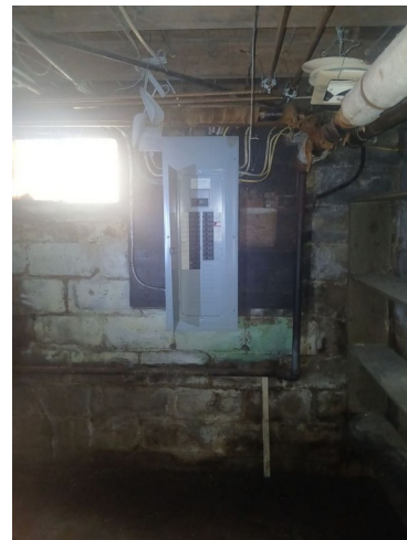
Figure 18. Electrical panels on block foundation wall (site photo 42)
