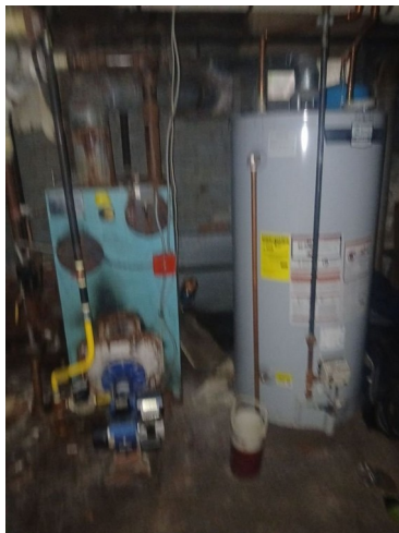
Figure 17. Boiler and tank water heater (site photo 31)
