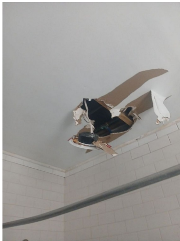
Figure 12. Bath ceiling opening (site photo 73)
