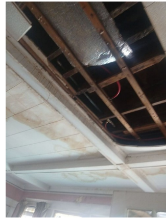
Figure 7. Open ceiling with framing, foil duct, stained tiles (site photo 15)
