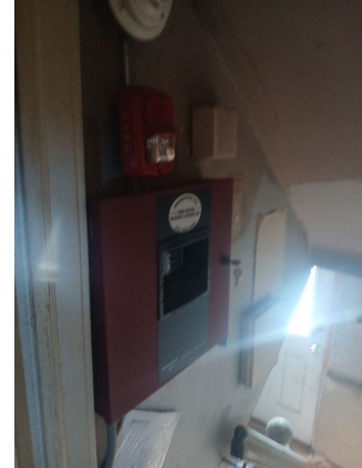
Figure 16. Fire alarm control panel (site photo 27)
