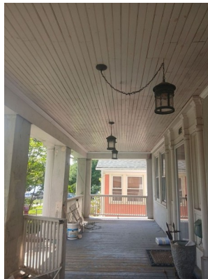
Figure 2. Front porch, beadboard ceiling (site photo 3)
