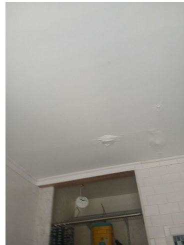
Figure 13. Bath ceiling bubbling (site photo 74)
