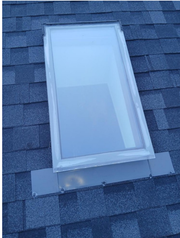
Plate 10 Skylight apron, exposed fasteners
