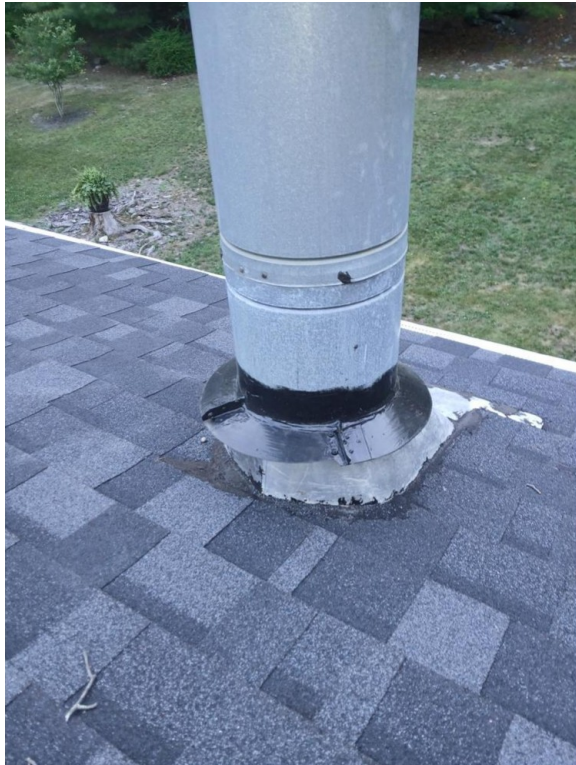
Plate 3 Base relies on surface cement
