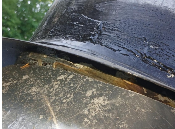
Plate 6 Unsealed flashing joint, close view
