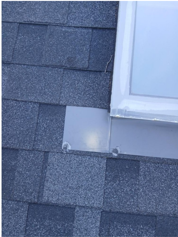
Plate 9 Skylight flashing, fasteners and lifted shingle
