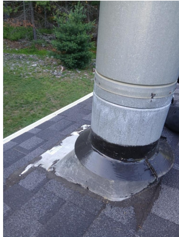
Plate 4 Collar tight, flashing beneath unsealed
