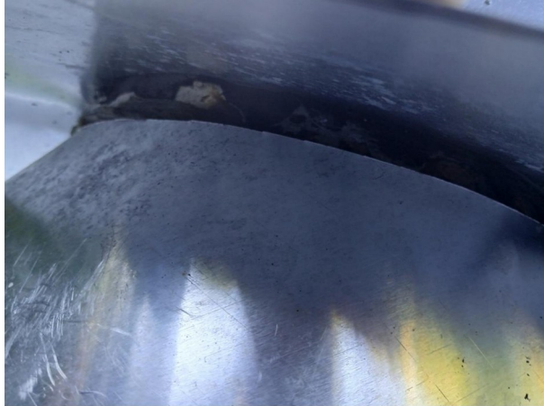
Plate 5 Unsealed flashing joint beneath the collar
